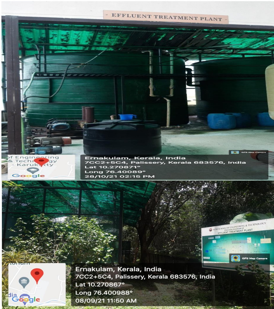
Effluent Treatment Plant installed within the campus with layout sketch
