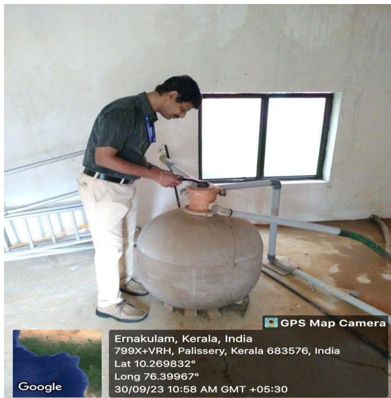
Bore well recharging installed in the Administrative Block
