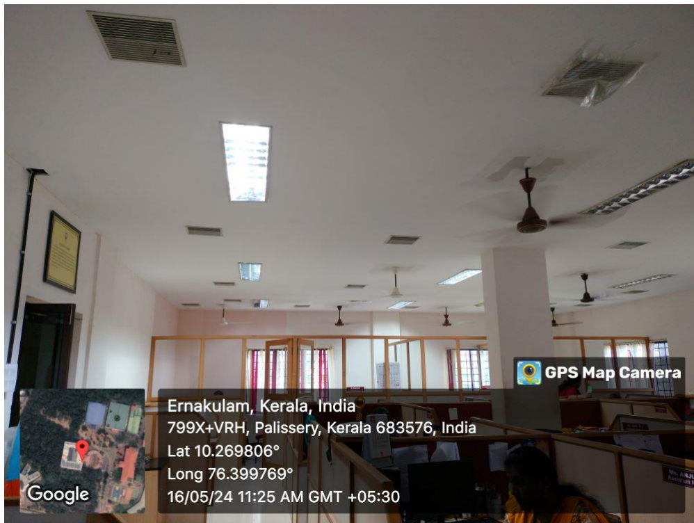
LED lights installed at the Department Staff rooms
