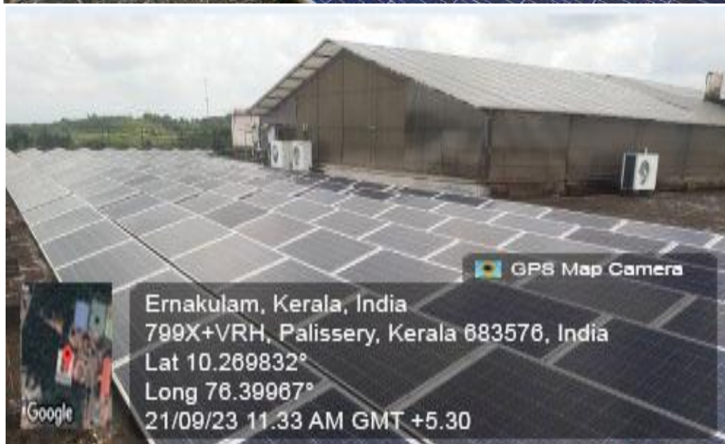
Solar Power Plant installed at the roof of Administrative Block
